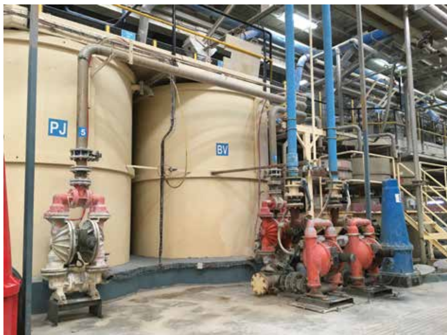
Image 1. Air-operated double diaphragm (AODD) pumps in operation at a ceramic plant in Spain (Images courtesy of PSG)
