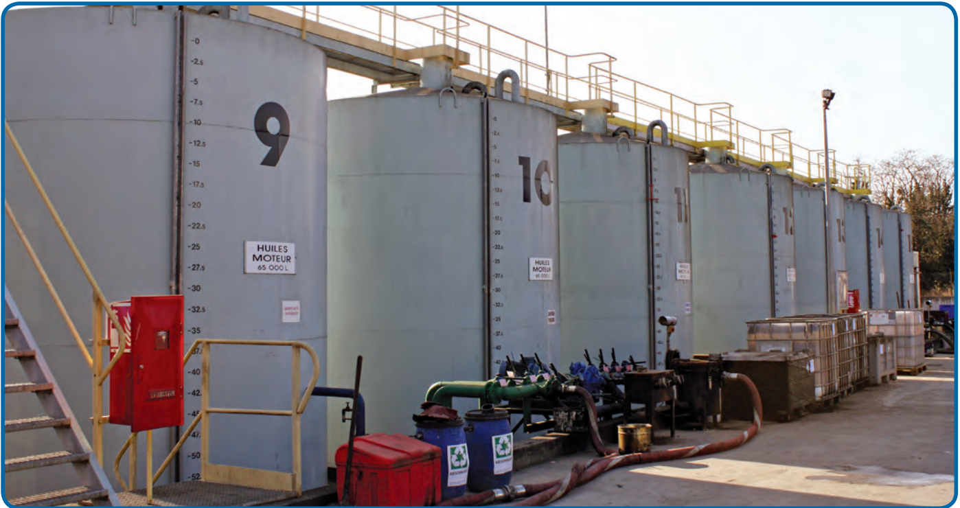
Mouvex A Series Eccentric Disc Pumps are also used within the storage tanks.
