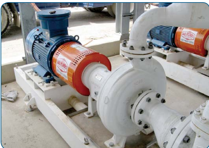
Griswold™ 811 Series centrifugal pumps with the 17-inch impeller were selected
