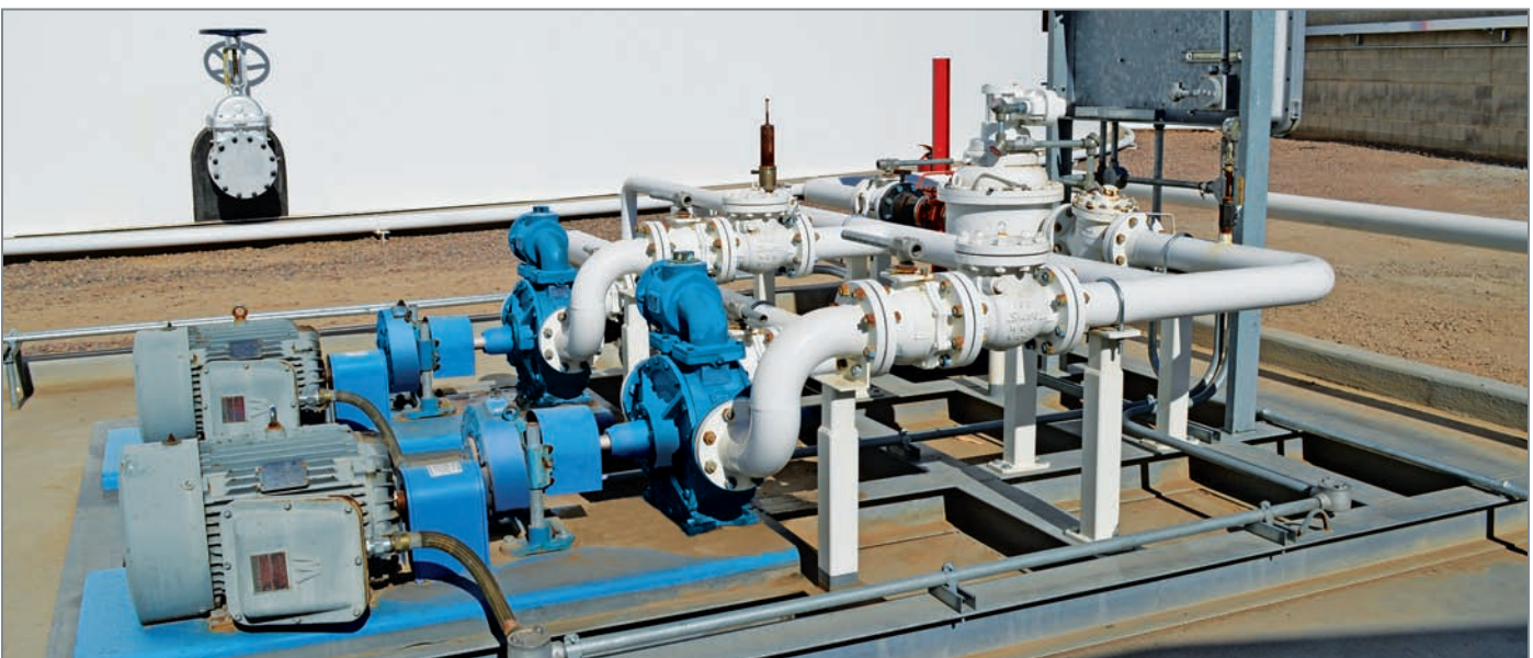
Among the many benefits that sliding vane pumps can offer to storage terminals are their ability to handle very-thin liquids along with those that have viscosities to 50,000 cSt.
