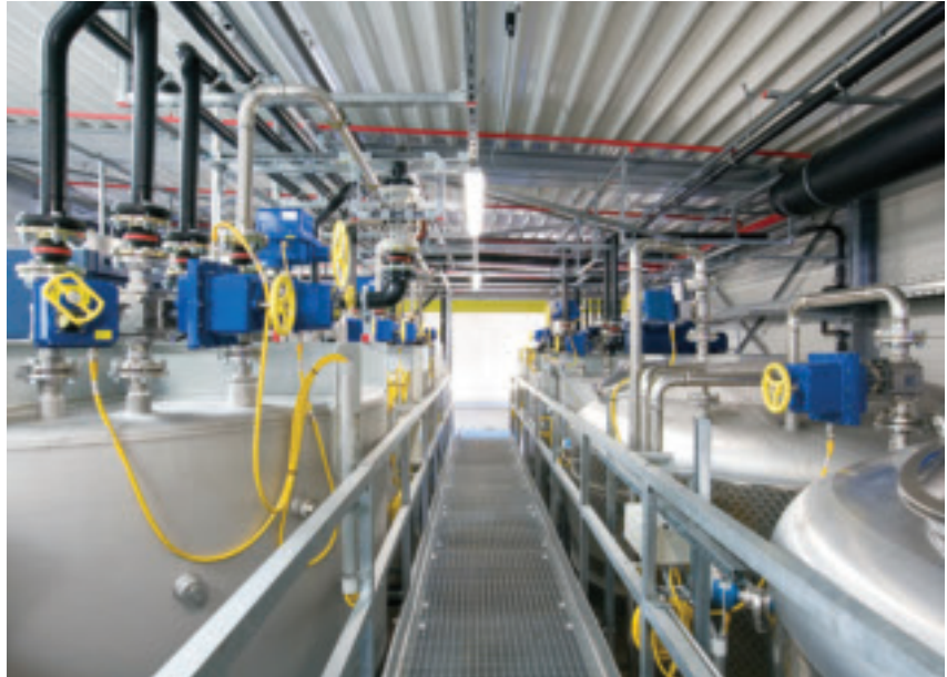
CRS designs, builds, installs, operates and maintains the reprocessing infrastructure at its customers' facilities to ensure a consistent, high-quality product at a low operational cost.
