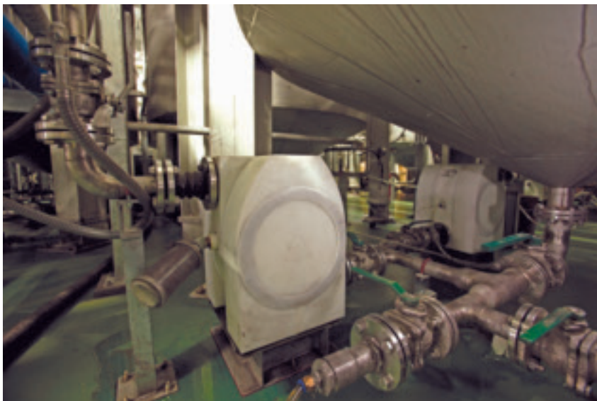
Almatec E-Series pumps installed at one of CRS Reprocessing Services' newest slurry reprocessing facilities in Korea.
