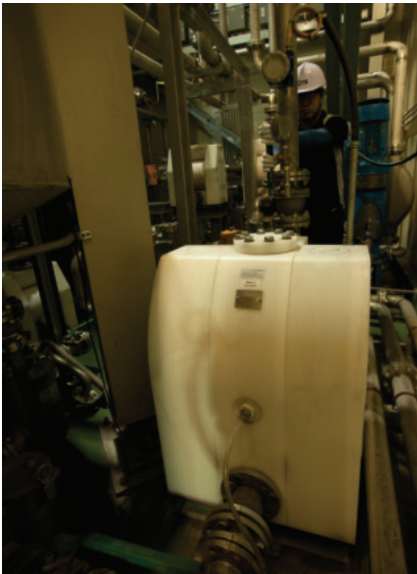
Almatec E-Series pumps have reduced CRS's maintenance costs by roughly 80% versus other pumps.
