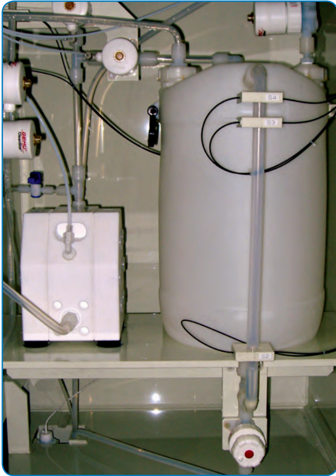
Wet Benches circulate and supply etching media such as acids and caustic fluids in a solar wafer manufacturing facility. Photo courtesy of S.P.M. srl, Italy.
