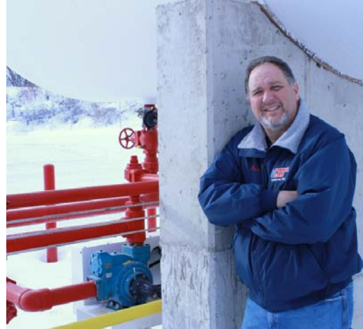
Greg PirkI stands next to one of the Blackmer® 3-inch LGL sliding vane pumps installed during his bulk plant upgrade.
