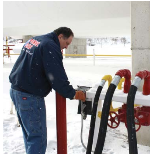
Greg Pirkl activates the shutoff valves at his recently upgraded bulk plant.
