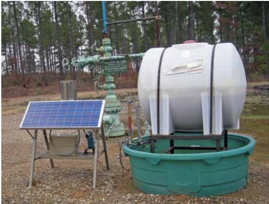
A solar injection powered system installed at a wellhead site.
