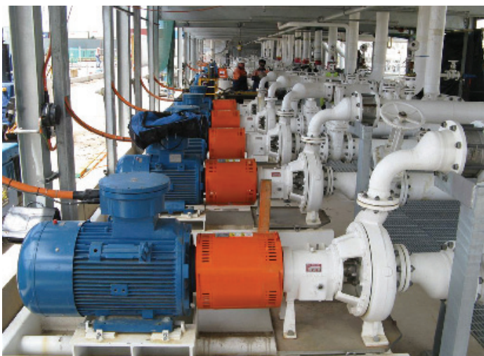
Pumps are the heart of any storage terminal operation. Proactive preventive maintenance is critical for optimum performance
