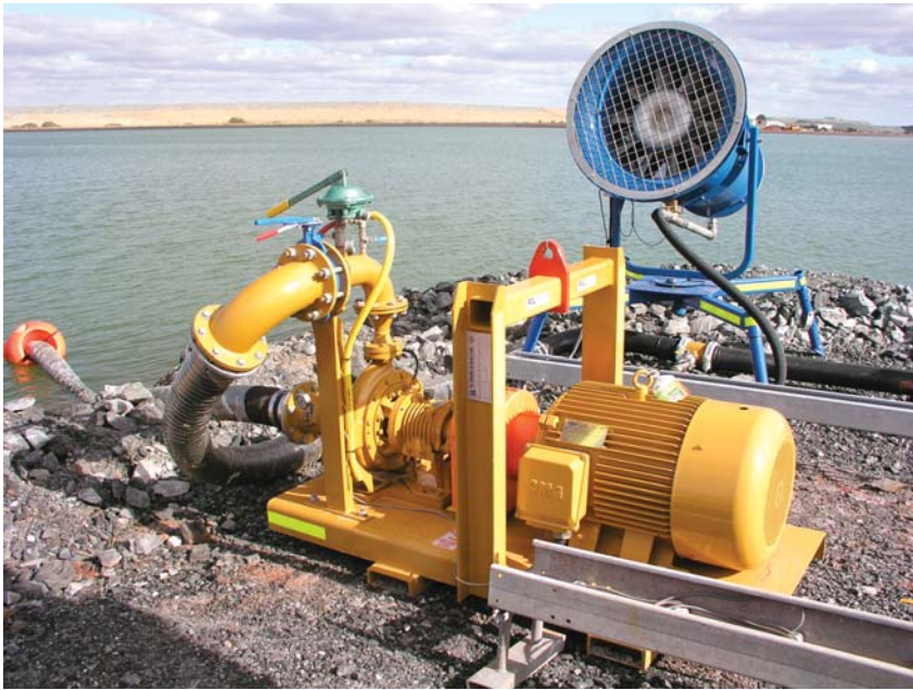
Evaporative dispersal systems typically include one pump per every six evaporator units.
