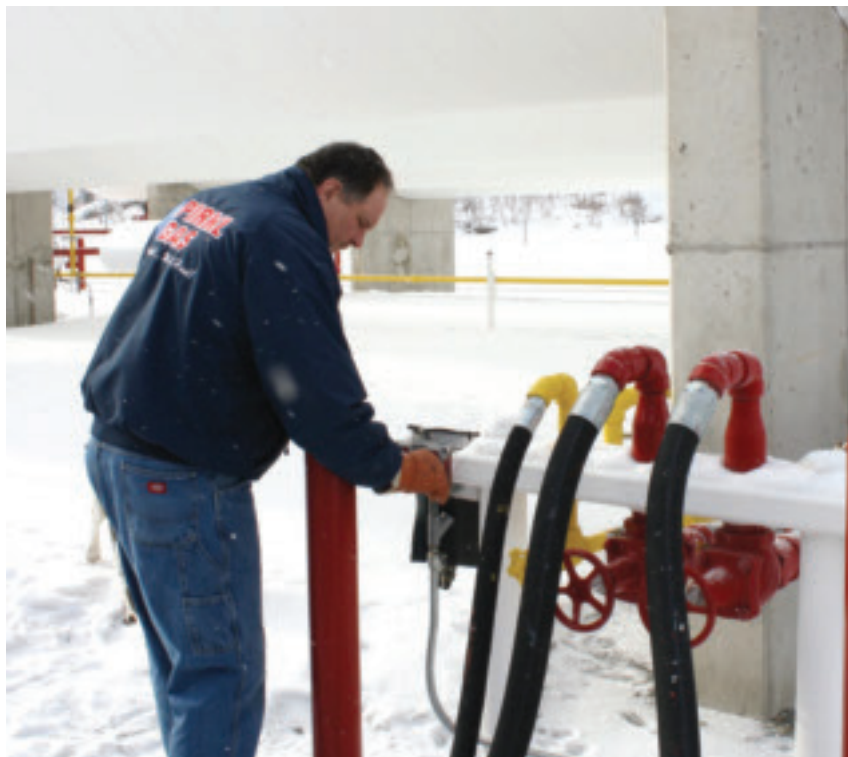
Figure 2. Greg Pirkl, president of Pirkl Gas Inc activates the shutoff valves at his recently upgraded bulk plant.
