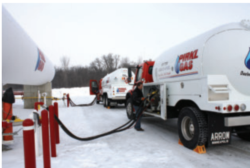
Figure 1. Since the installation of Blackmer 3-inch LGL sliding vane pumps overall loading times at the gas bulk plant are down from 40 minutes to 13 minutes on its 5,000 gallon (18,900 litres) trucks.
