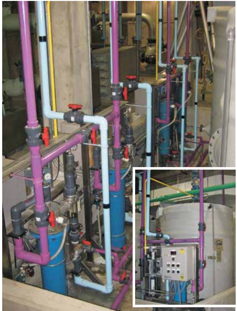
This system simplifies the polymer blending process because it has been designed to effectively activate all types of liquid polymer.
