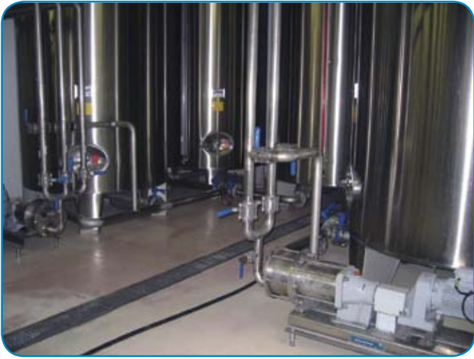
Figure 1: Mouvex eccentric disc pump in a transfer line from sweetener storage.
